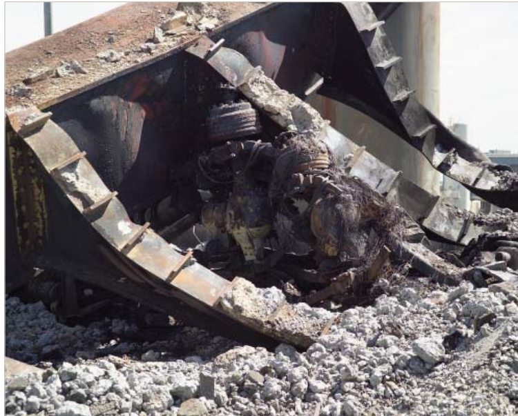
Remnants of the petroleum truck that exploded and destroyed the MacArthur Maze bridge are barely recognizable amid the rubble of disintegrated concrete and twisted girders.
